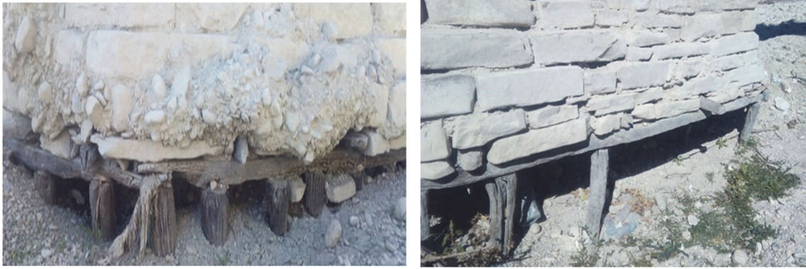
Fig. 4: Exposed wood piles of diameter 12-18 cm (IMK)
