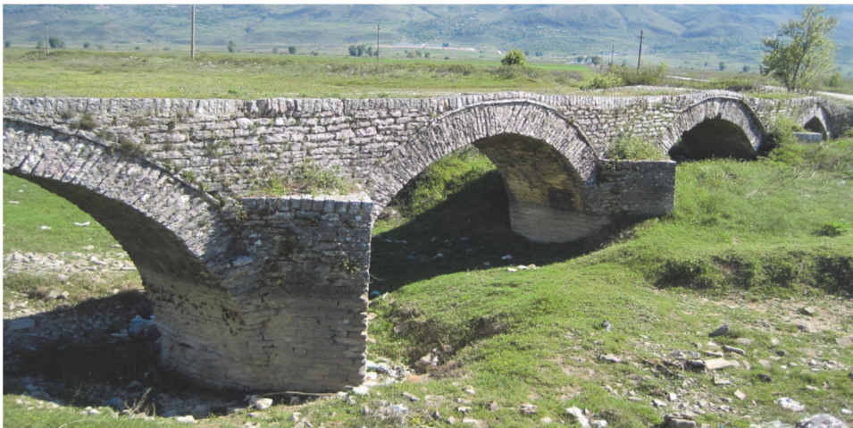
Fig. 1: Kollorcka Bridge pier scour in the dry period of the year
